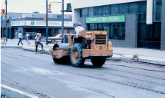
Figure 5. Compaction of the base is essential to all flexible pavements including those built with concrete pavers.
