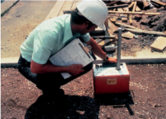
Figure 6. Monitoring of base compaction during construction minimized the likelihood of settlement later.
