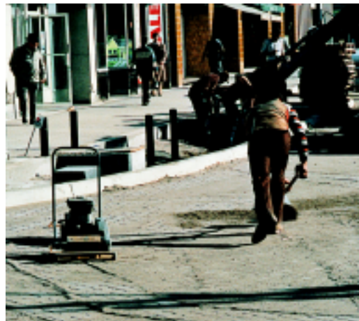
Figure 11. Sand swept into the joints and compaction of the pavers transform the pavement from a loose collection of units to an interlocking load-bearing pavement system.
